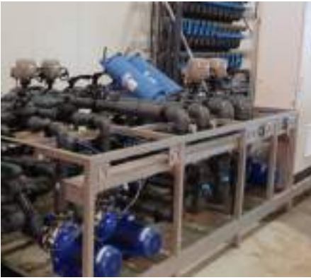
Photo left: installation for underground heat storage at Duijvestijn Tomaten (©Trees Borkus Henskens)
