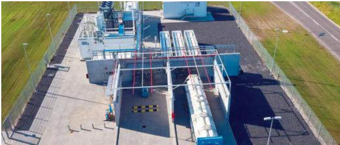
Fig. The Cummins PEM Electrolyser in Denmark, Europe. Source: https://www.3blmedia.com/News/Cummins-PEM-Electrolyzer-Will-Supply-Hydrogen-Denmark-Europe-Demonstrating-Strong-Hydrogen
