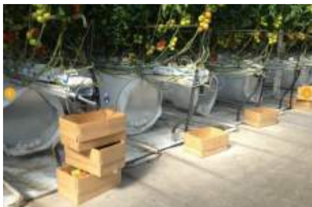
Fig. The air distribution sleeves in the Ultra-Clima greenhouse from KUBO, at D’Vine Ripe in South Australia.
