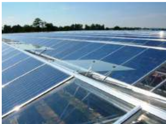
Hortisolar panels in Italy, solar roof, 2MW.
